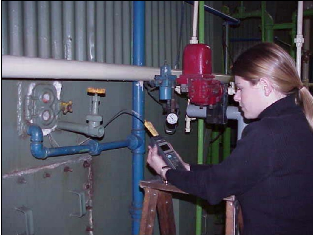
Fig. 10, Furnace temperature measurement system
