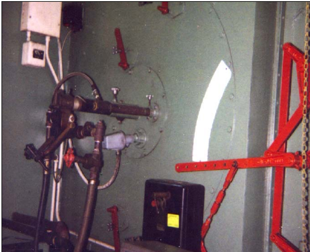
Fig. 4, Burner nozzle for the No. 2 boiler
